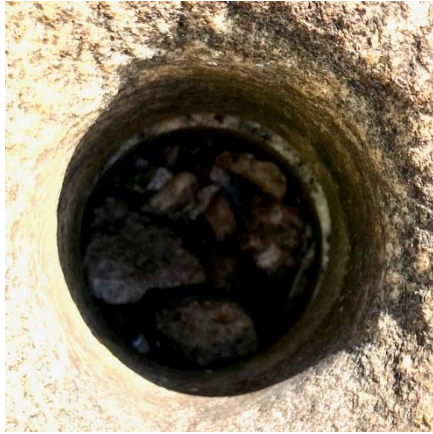
Figure 2-borehole near the center of the lens of rock that detached around June 14, 2024. The ledge visible in the upper right portion of the hole, about 5 inches down, is the separation surface, and shows that the lens moved very slightly (and counterintuitively) opposite to the surface slope."
